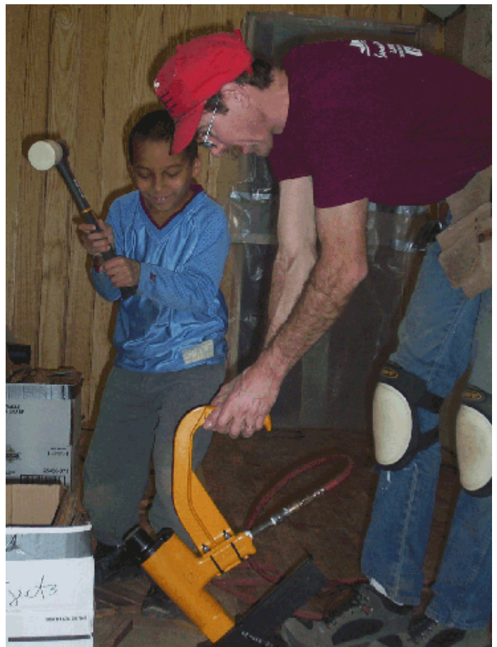
Caleb and Glenn working hard on the new floor at Sky-Vue Lodge
